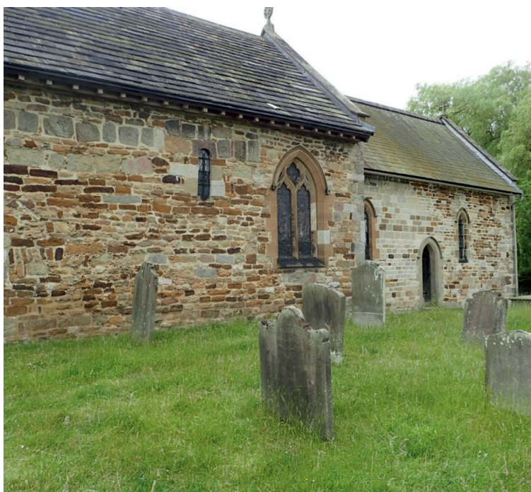
Fig. 4 St Michael's Church, Crambe. The stonework of the nave (left) was pointed with NHL 2.0 six months before the chancel (right) was repointed by ourselves with lime-rich hot-mix mortar. It is reasonable to say that the chancel fabric is now drier than that of the nave.
